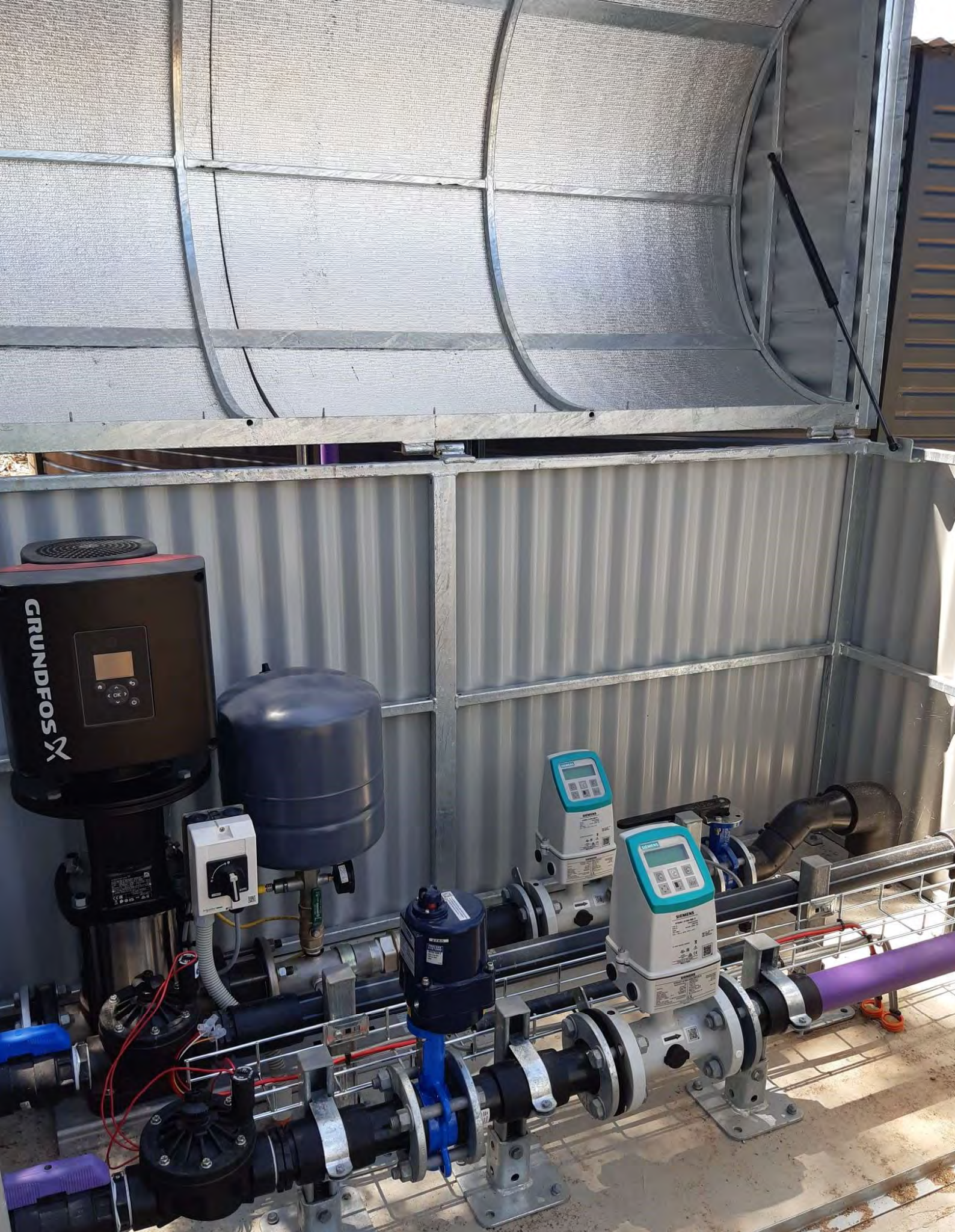
Pump station equipment, Ladywood Reserve, Modbury North
