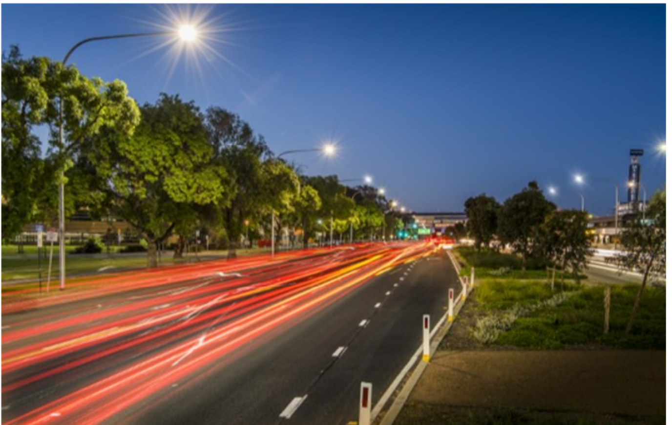
Public street lighting, while an essential service, is one of the largest energy uses in the city.
