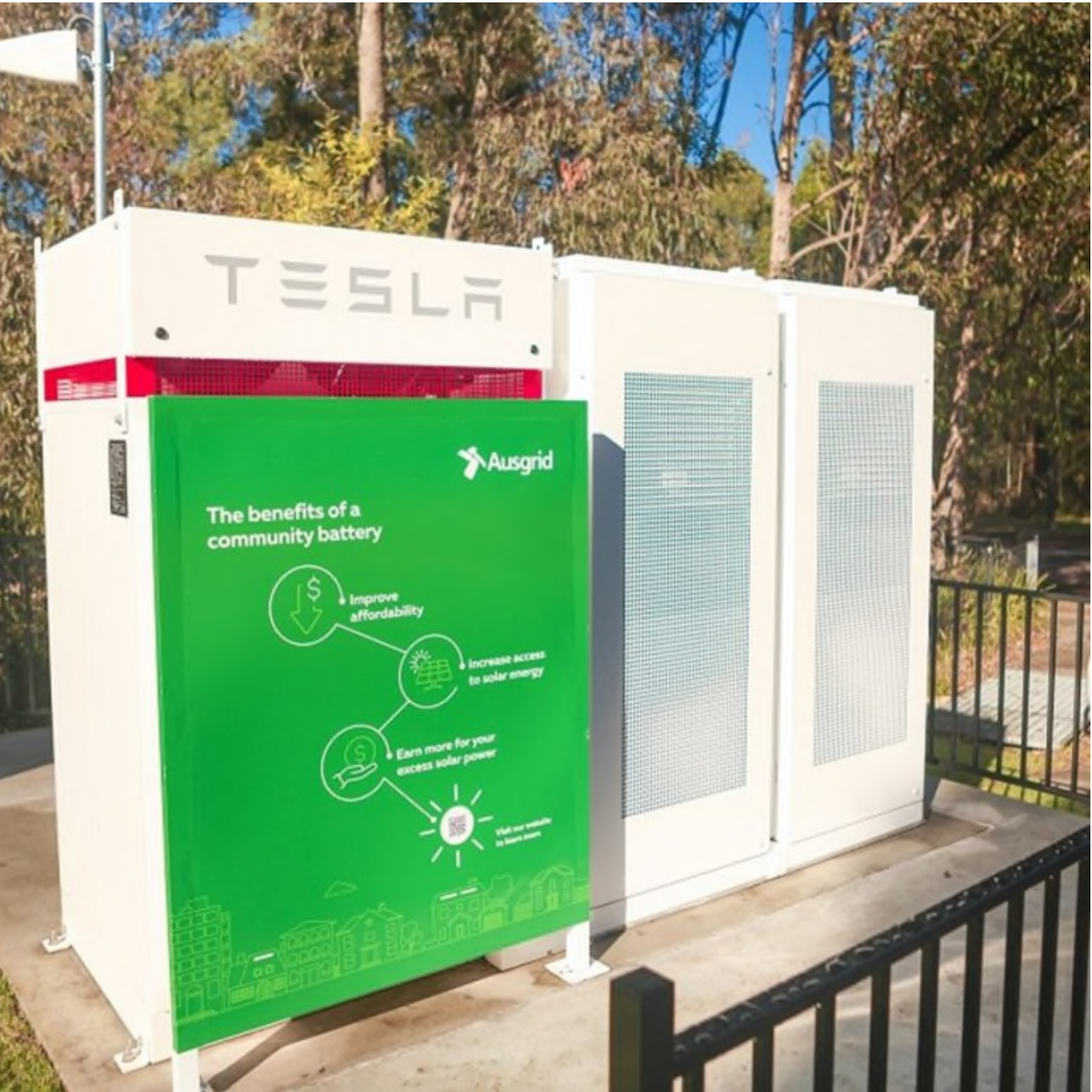
Small-scale battery energy storage systems (BESS) and ‘community batteries’ offer the capability to store electricity when it is surplus and cheap for use later when it is in high demand.
