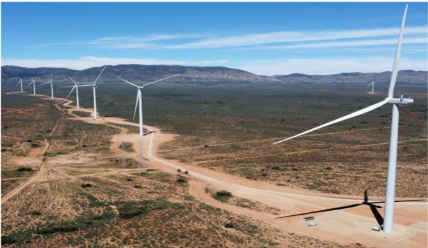
Wind generates almost half of the electricity used in South Australia. The Goyder Wind Farm supplies electricity to Council through a power purchase agreement.
