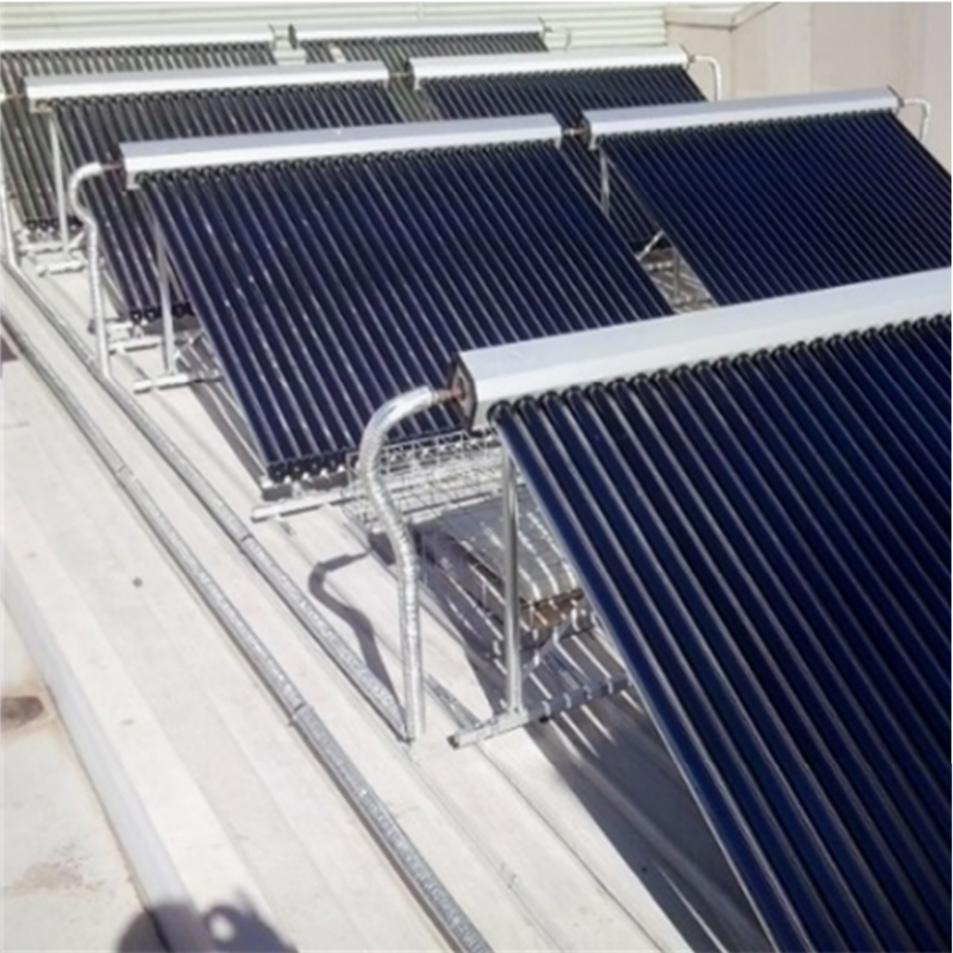
Solar thermal water heaters at Golden Grove Recreation and Arts Centre. Solar water heaters are an efficient method of heating water and have been used in domestic and commercial buildings in Australia since the 1950s.
