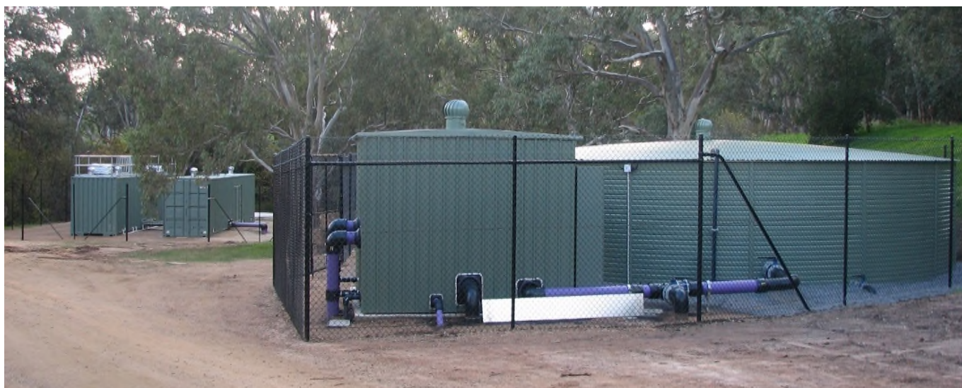
The water treatment plant at Wyn Vale Dam treats stormwater, which supplies Council's ASR schemes.
